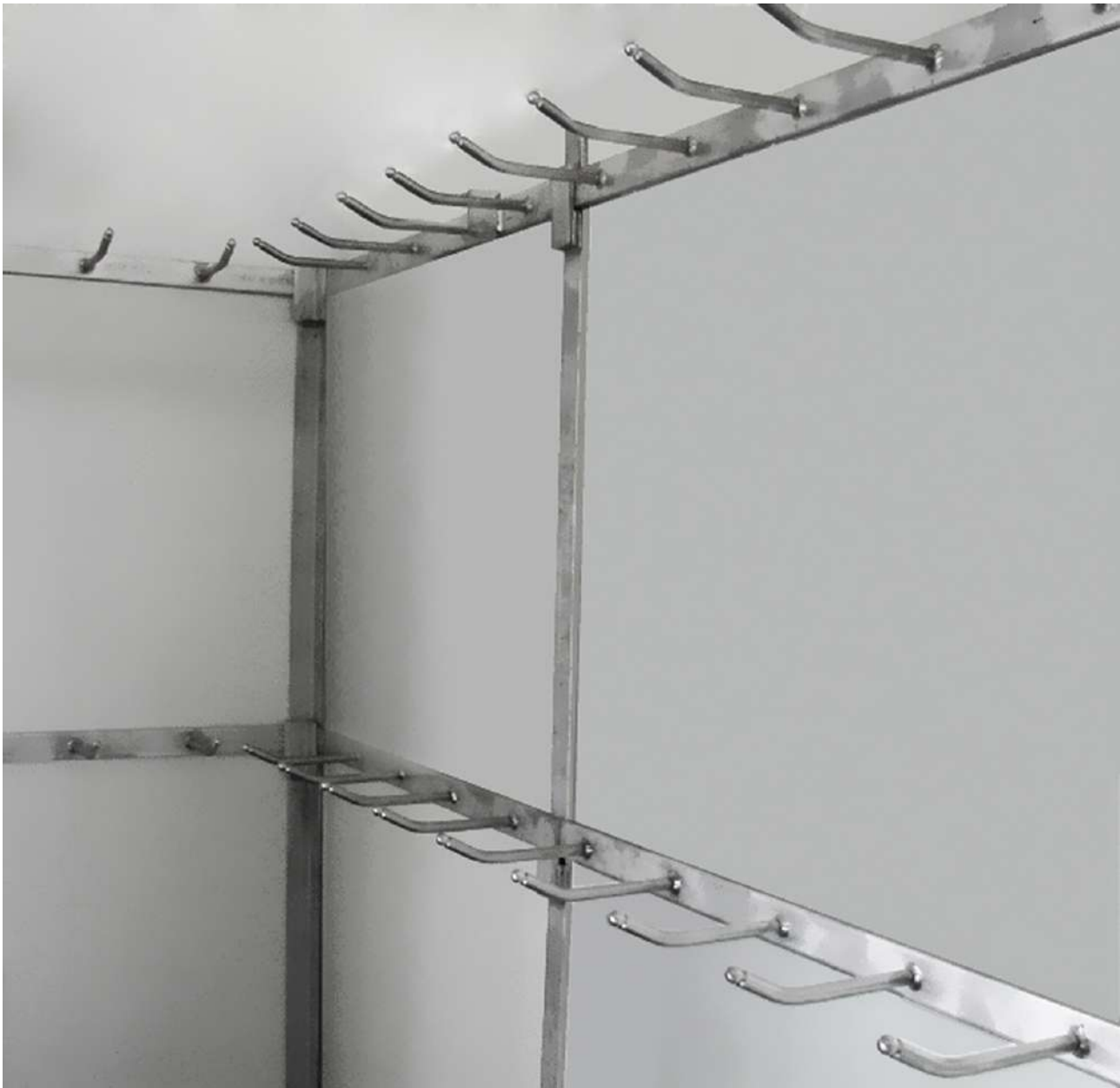
Inox hooks inside a cold room for meats
